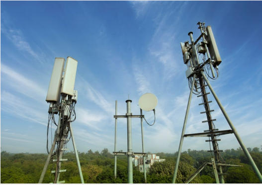
Indian telecom towers
